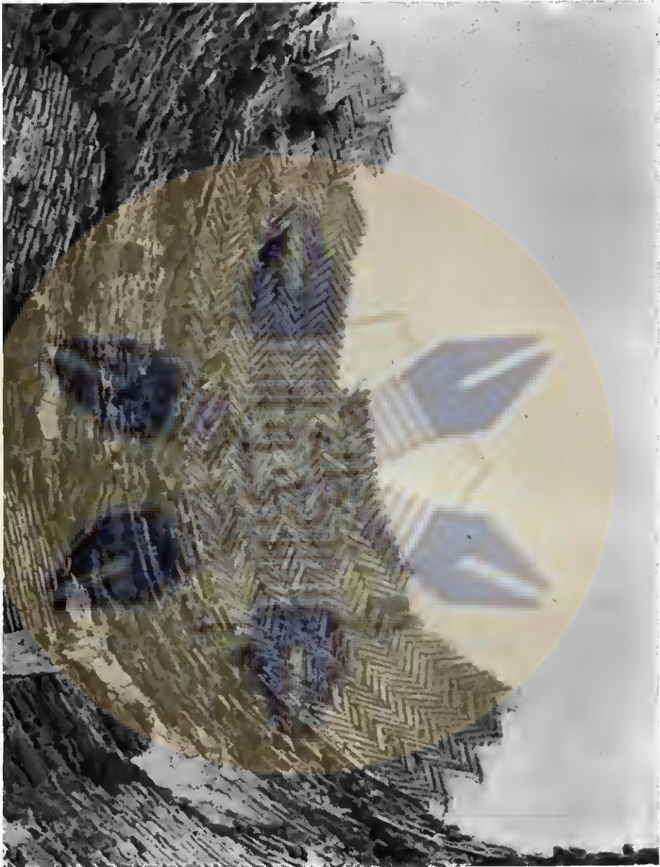
109. Tomb of king Fateh Khan's sister. Interior view of galf collapsed dome showing bricks used in zigzag pattern for strength as well as to construct curved surface.
